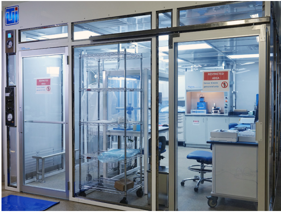
NKC ISO 7 Clean Room
